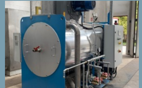
Gurit Carmignano (Italy) installed a new steam generator which achieved a saving of up to 3m3 heated water per day, also reducing energy use
