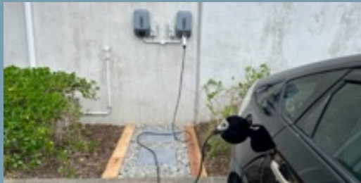
Installation of E-car chargers for staff to use during the working day
